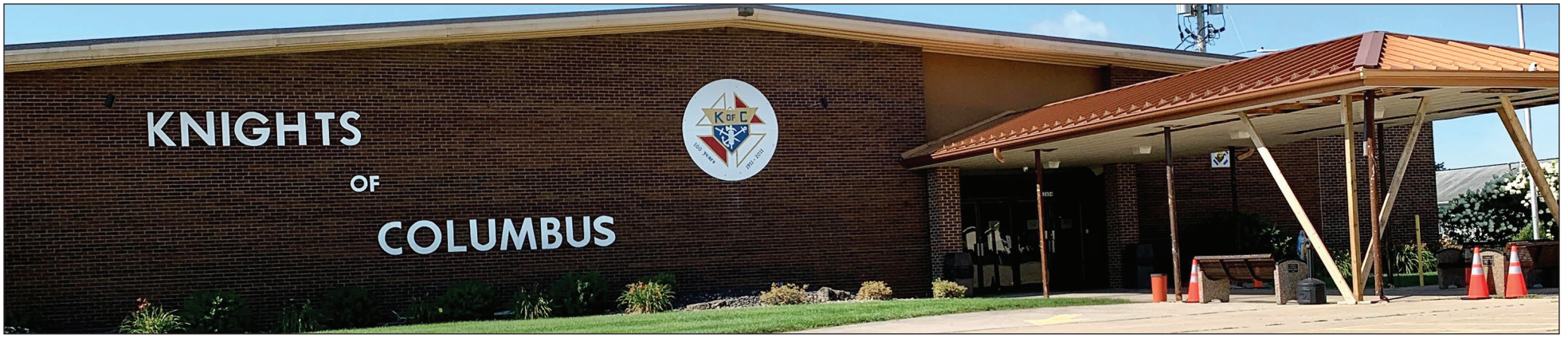
The Columbus Club is working on repair of the front awning at the entrance of the hall. It has been properly braced so that work can continue and the structure can be safely repaired for future functions.
